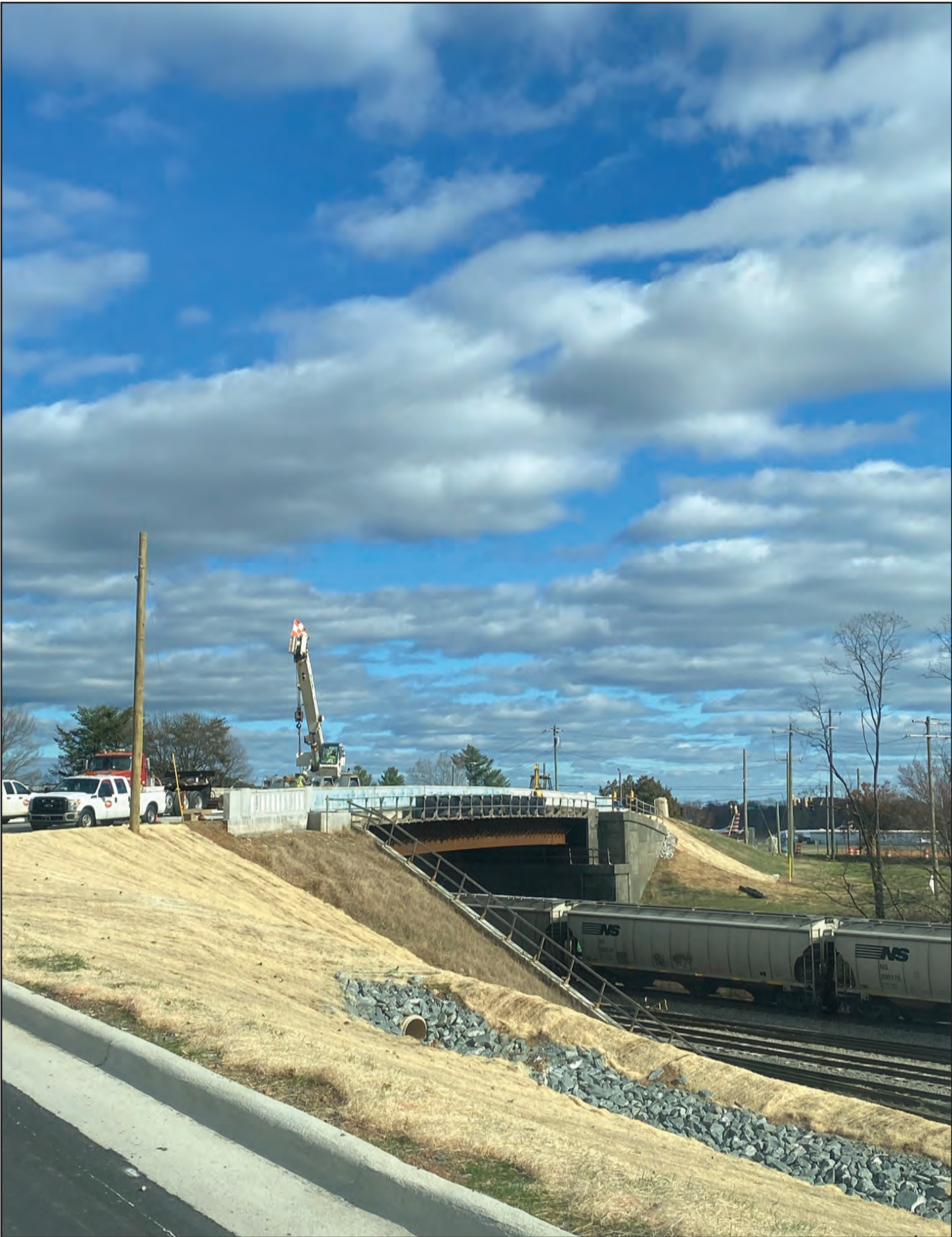
Akron Drive replacement bridge over railroad at North Liberty Street nearing completion
